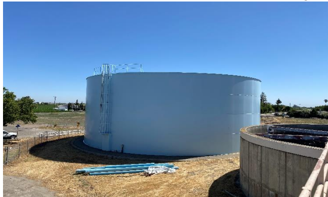
Figure #4: Existing ground level storage tank.
