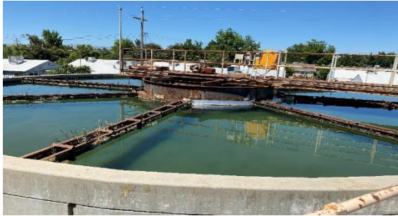
Figure 3: California Aqueduct water in the Dos Palos water treatment plant clarifier.
